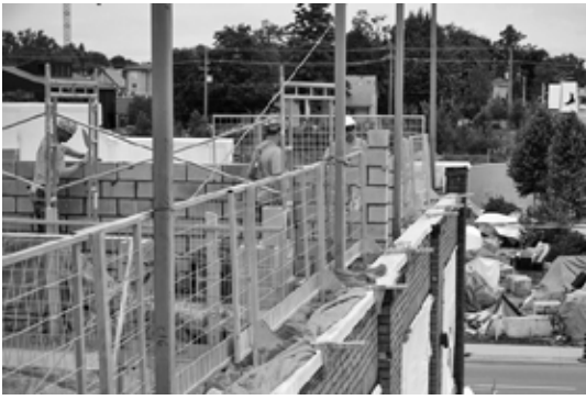
Construction of the new third floor that will include 22 units of housing
