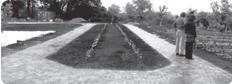
One of the interlocking brick pathways gleaming after installation with first crops starting to grow.
