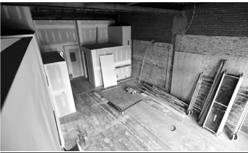
Photo of the construction of the top floor apartment at 58 Queen that has now been turned into a four bedroom family-sized apartment
